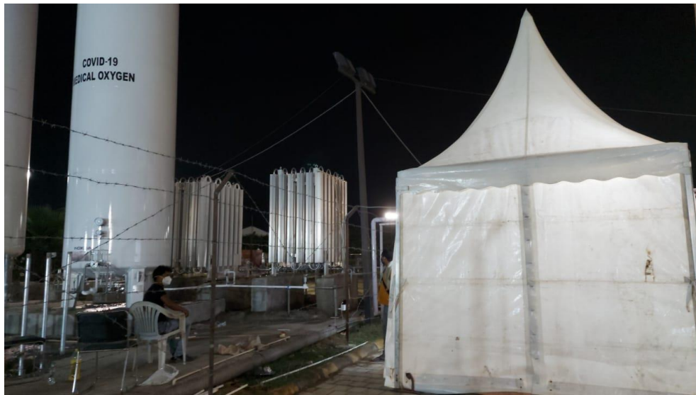
Photo 5.3: OXYGEN plant (40 KLD) installed at Atal Bihari Vajpayee COVID Care Hospital, Lucknow, Uttarpradesh
